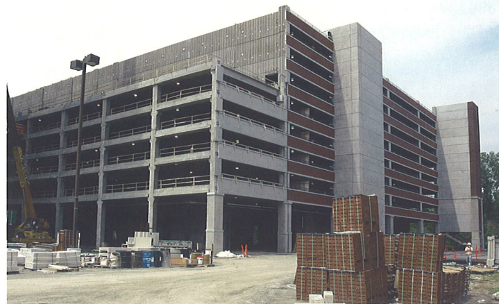
THE REAR OF THE 2350-PARKING SPACE GARAGE. THE FIFTH FLOOR WILL FEATURE A POOL AREA WITH LANDSCAPED GROUNDS AND WATERFALLS.
