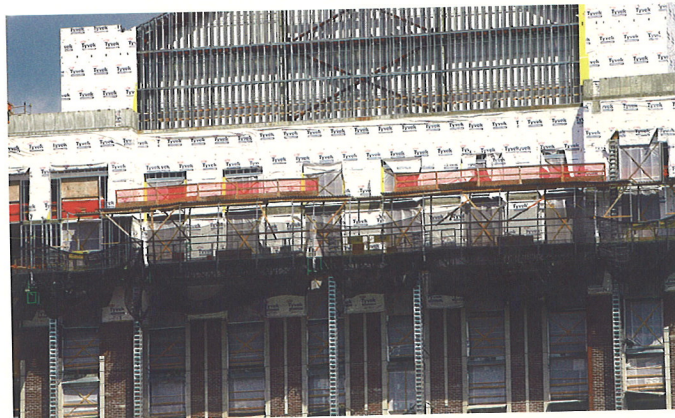
CORRUGATED STEEL PROVIDES A CANOPY TO PROTECT THE WORKERS FROM FALLING DEBRIS WHILE NETTING BELOW THE PLATFORM PROTECTS PERSONS ON THE GROUND.
