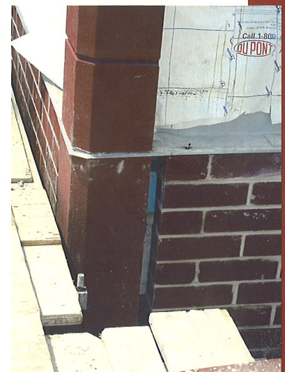
GFRC WAS SPECIFIED AS A LIGHTWEIGHT ALTERNATIVE TO PRECAST CONCRETE. HERE, A 2-IN. CONTROL JOINT IS VISIBLE.
