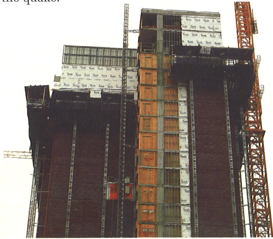
HYDRO MOBILE SCAFFOLDING PROVIDES A SAFE WORKING ENVIRONMENT WHILE HELPING TO SPEED THE PROJECT ALONG.
