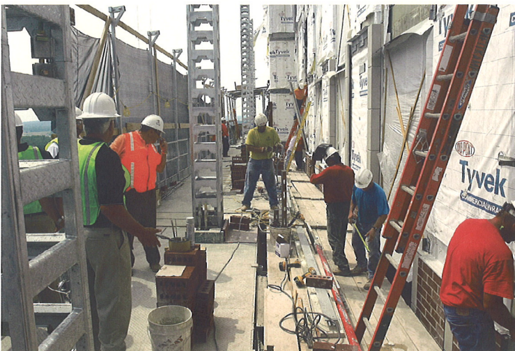
TWO HUNDRED FEET ABOVE THE MISSOURI RIVER, WORK ON THE HOTEL'S EXTERIOR PROCEEDS IN SMOOTH PRECISION.
